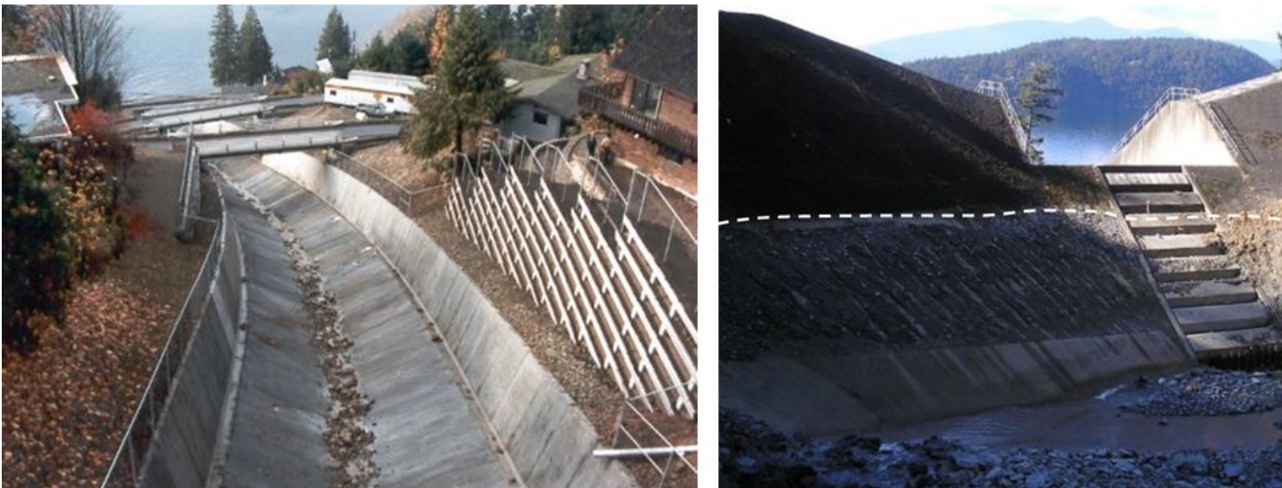
Figure 7.3.5 Two strategies for mitigating debris flows in western Canada. Left: A concrete-lined channel along a creek allows debris to flow quickly through to the ocean. Right: A debris-flow catchment basin along a creek. In 2010, a debris flow filled the basin to the level of the dotted white line.
