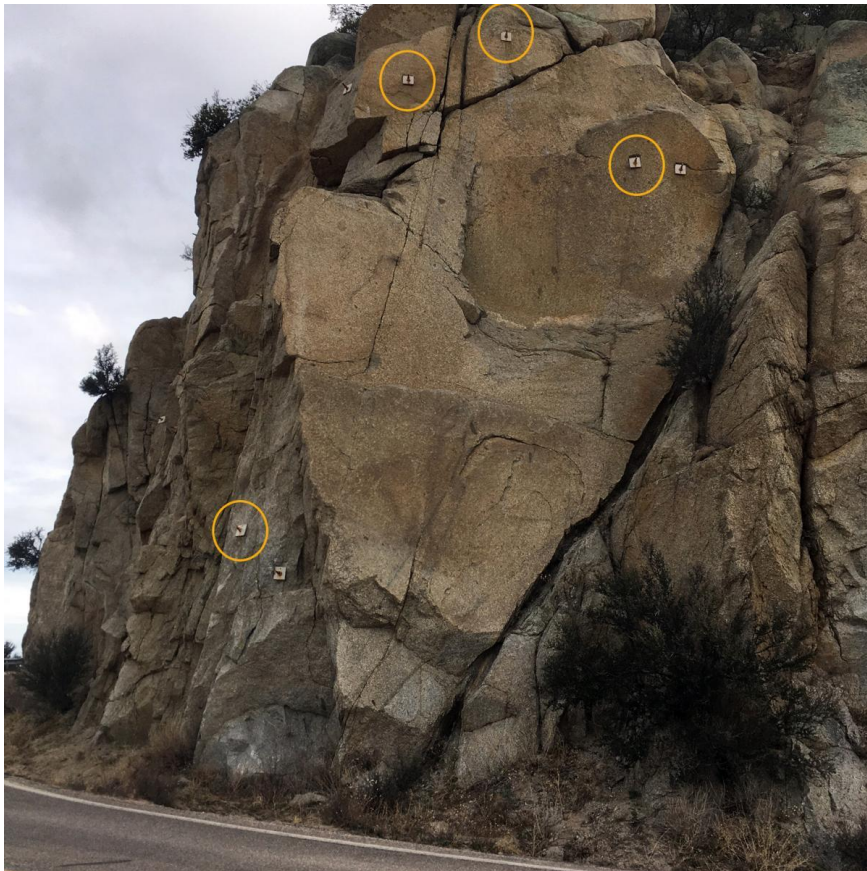
Figure 7.3.1 Bolts are used to keep rock face in place. Kitt Peak, Arizona. M. Conway, AZGS
