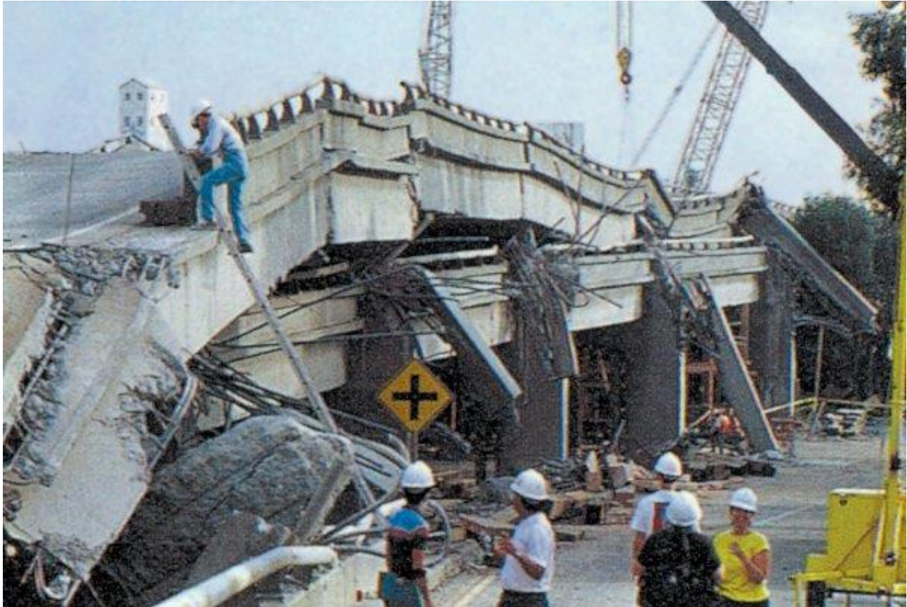
Figure 5.4.2 The Cypress Structure, the freeway approach to the Bay Bridge from Oakland, collapsed during the Loma Prieta earthquake, killing 42 people. USGS , Public Domain .
